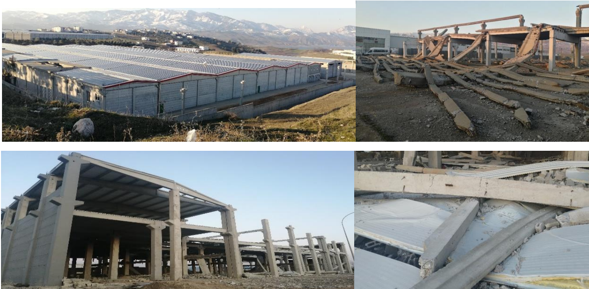
Figure 5.6. Overview of precast industrial building connection damage in Kahramanmaraş
