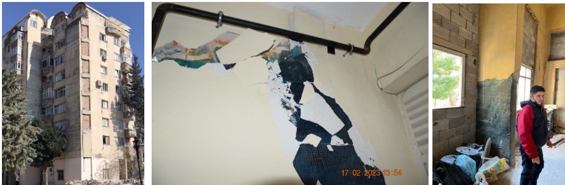
Figure 5.10. Performance of the strengthened building in Hatay
