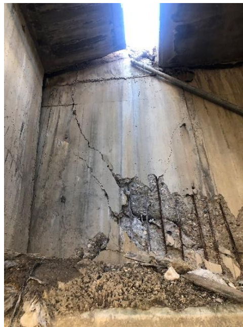
Figure 6.7. Abutment wall concrete spalling
