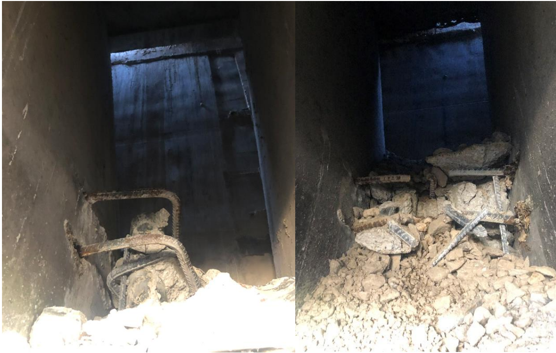
Figure 6.6. Shear key damage
