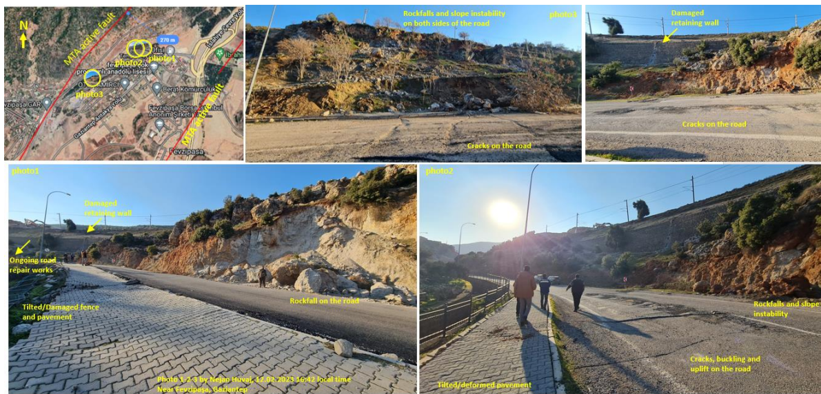
Figure 8.9. Landslides, rockfalls and surface cracks on the roads, near Fevzipaşa, Gaziantep causing disruption in the service (Active fault data from Emre et al. (2013)).
