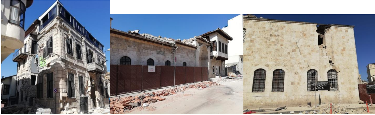
Figure 5.9. Damage in masonry structures
