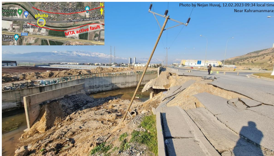
Figure 8.5. A landslide and crack/damages on the road next to a water canal, causing significant lateral displacement of a concrete retaining wall (pushed towards the water canal), a tilt on an electric pole, in southern part of the city of Kahramanmaraş (active fault data from Emre et al. (2013)).
