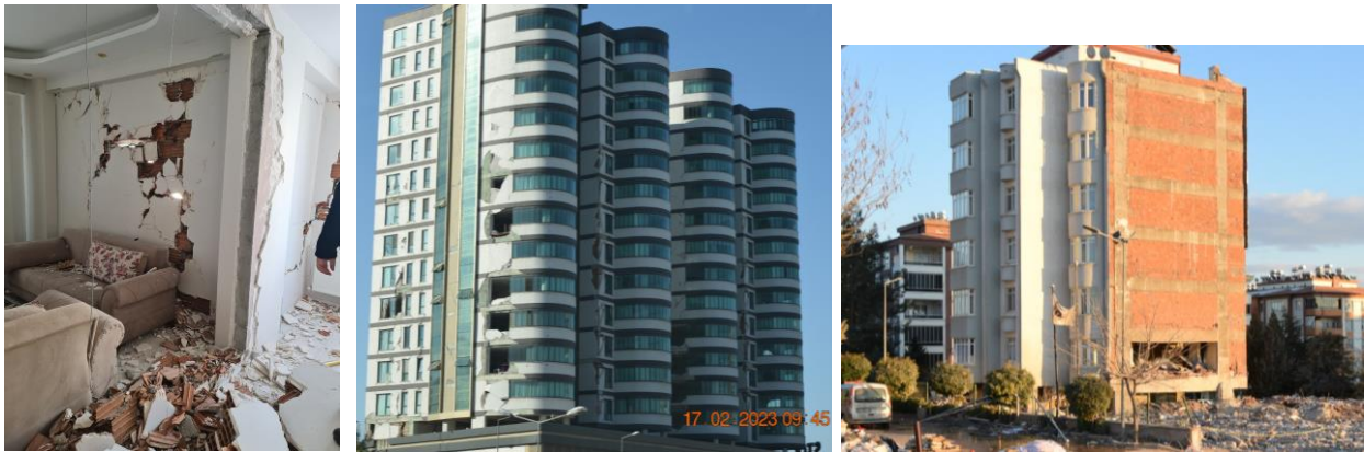
Figure 5.8. Infill wall damage examples
