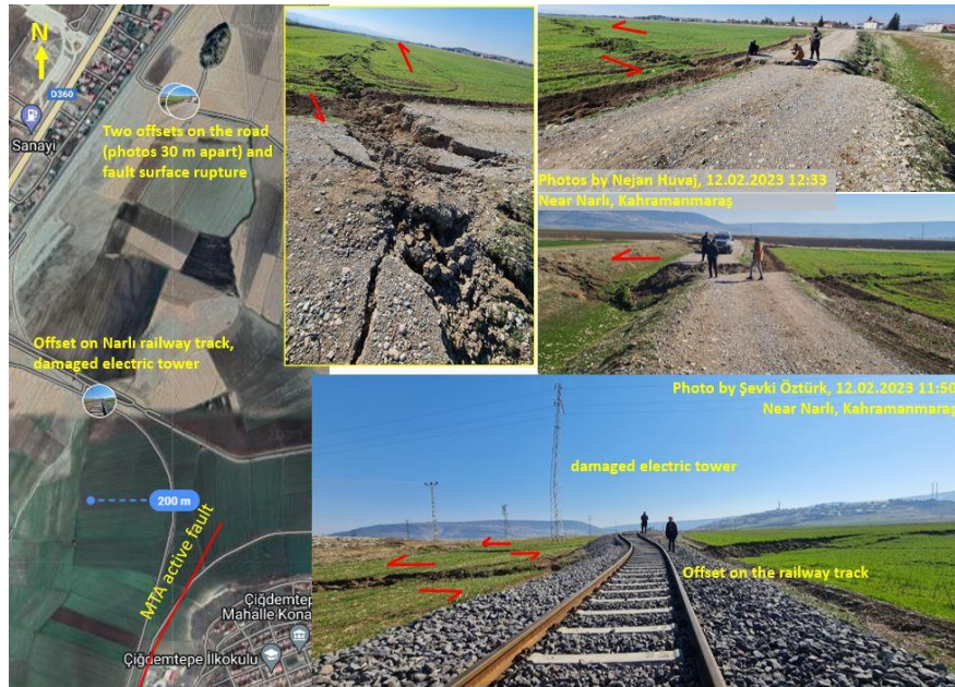
Figure 8.4. Surface rupture, offset, cracks and damages on railway tracks and roads, as well as a damaged electric tower, near the surface rupture (Narlı, Kahramanmaraş). (Active fault data is taken from Emre et al. (2013)).
