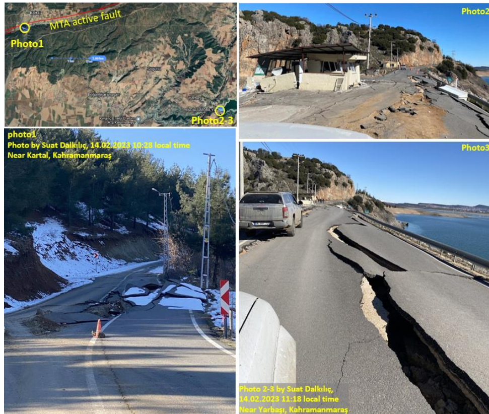
Figure 8.8. Landslides and surface cracks on the roads, near Kartal and Yarbaşı, Kahramanmaraş (Active fault data from Emre et al. (2013)).
