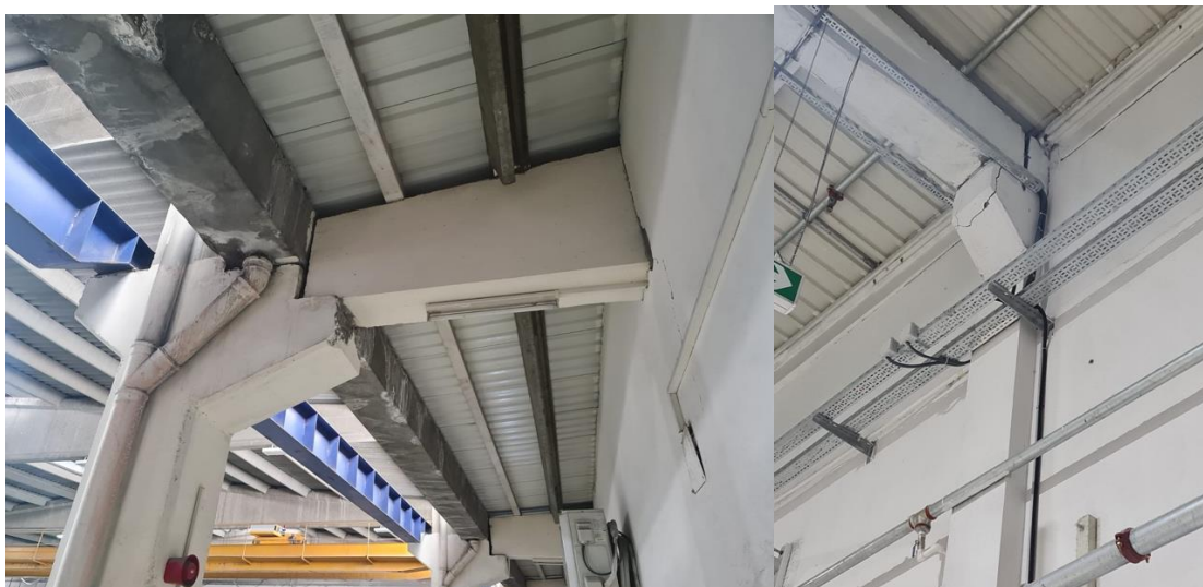
Figure 5.7. Corbel damages in Gaziantep
