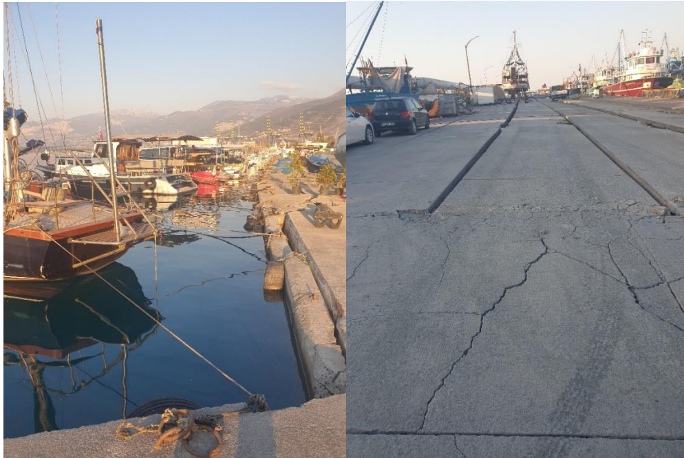
Figure 7.4 Structural damage at İskenderun Fishery Port
