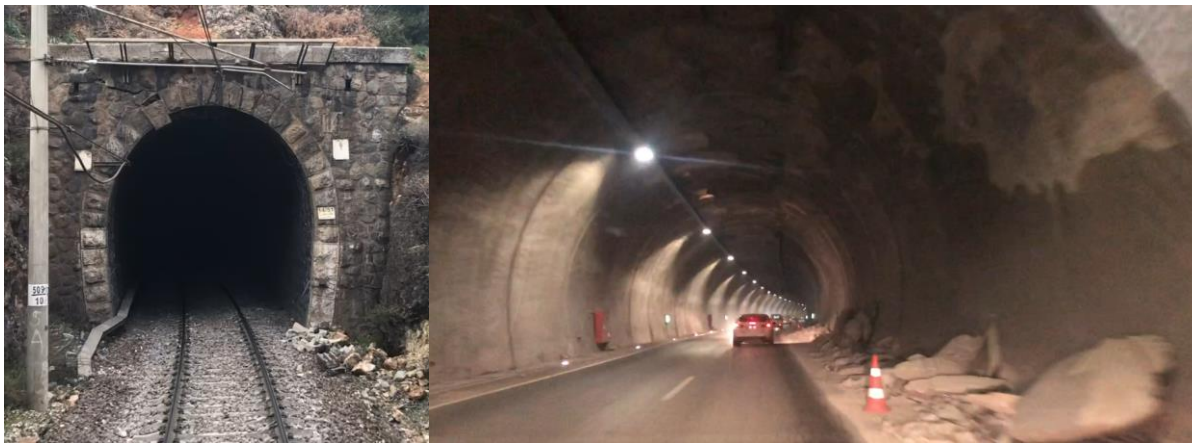
Figure 6.9. Tunnel portal movement and concrete spalling
